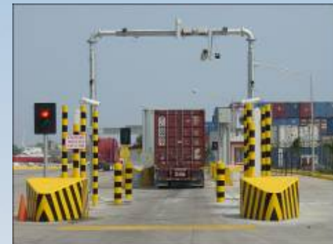
Megaports installation in Honduras
